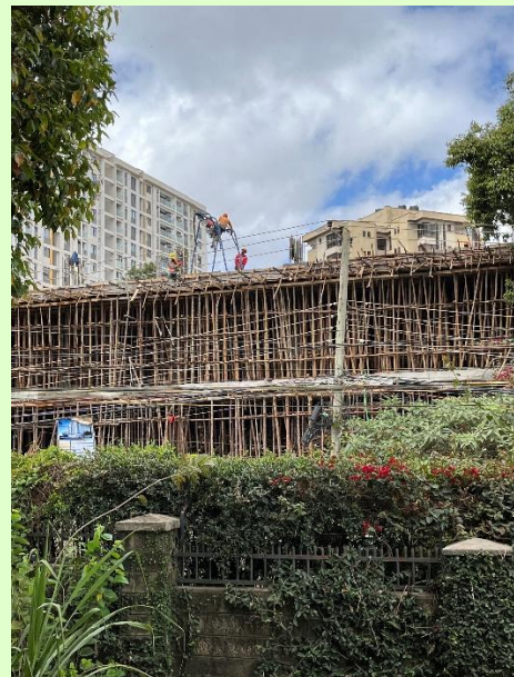
Construction site without safety measures
