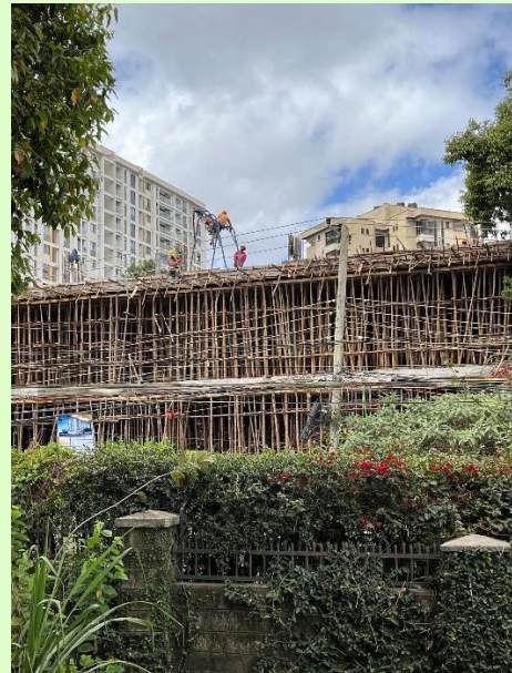
Construction site without safety measures
